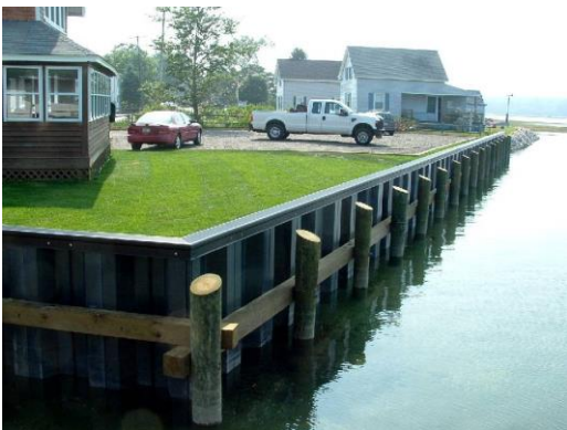
Hardened bulkhead shoreline in Scarborough, ME. Source: Maritime Construction and Engineering, LLC
