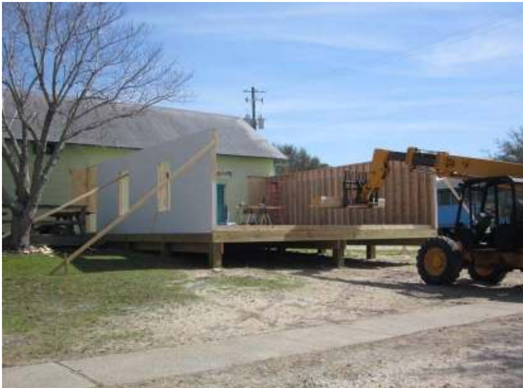
The facilities crew built a new classroom on the Endeavor building for the Discovery Hall Program.
