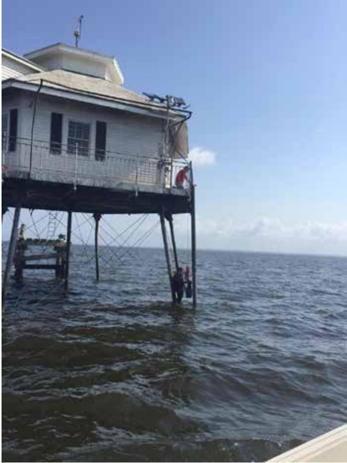
Yantzee Hintz and Hunter King working to repair damage done to the Middle Bay Lighthouse station that displays near real time data at www.mymobilebay.com . Data is transmitted to National Data Buoy Center (NDBC) and Gulf of Mexico Ocean Observing Systems (GCOOS) within thirty minutes of harvest.
